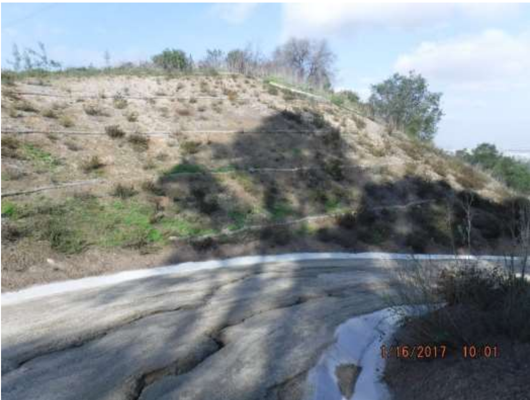
Figure 6: Erosion of access road at Tower 49-T12, Segment 8 Overhead. Photo courtesy of SCE.
