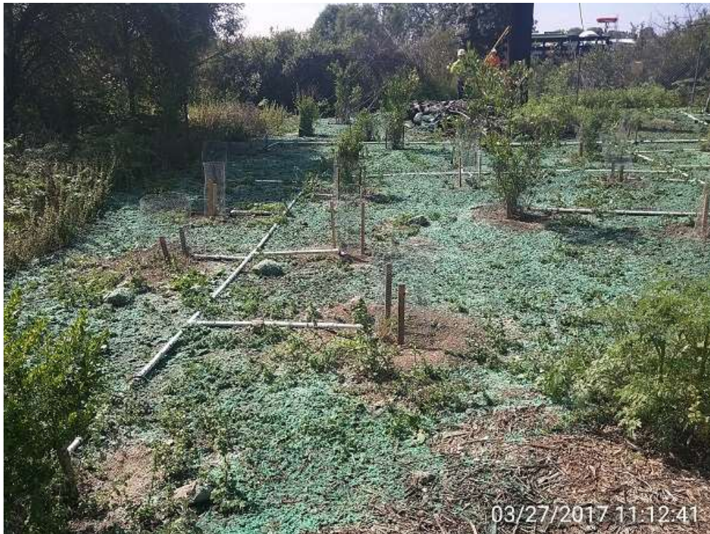
Figure 4: Restoration Site R003 after weed abatement and hydroseed activities, Segment 8. Photo courtesy of SCE.
