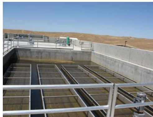
Cal-Water Bakersfield Surface Water Treatment Facility
