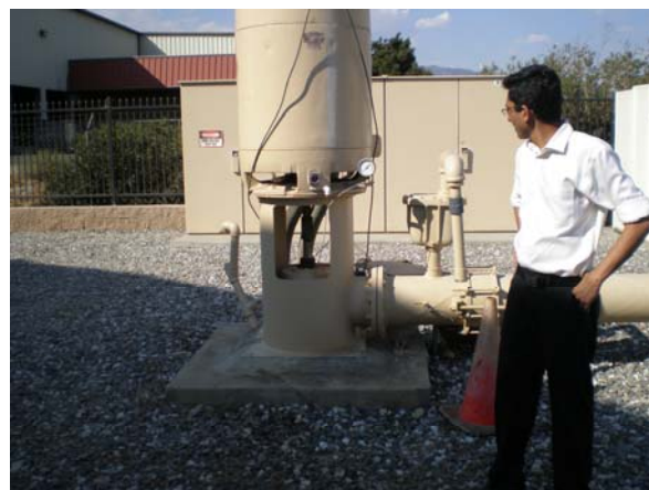
DRA engineer Nihar Shab inspects a San Gabriel well pump located in Fontana, California
