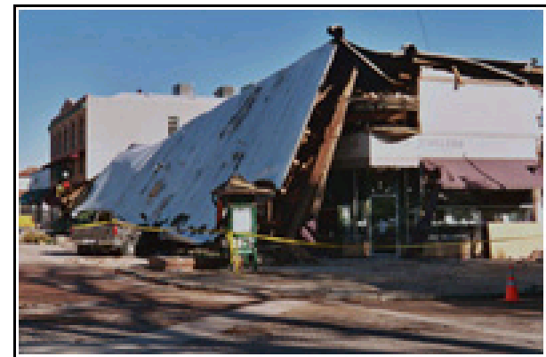
Paso Robles, CA January 25, 2004 -- Structures and a vehicle damaged in downtown Paso Robles in the 6.5 San Simeon Earthquake. FEMA Photo/Dane Golden
