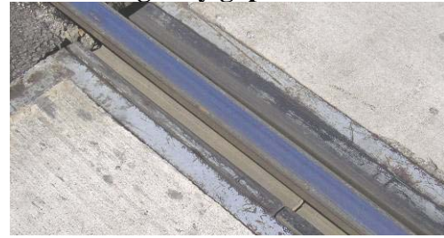
Figure 25. Flangeway gap with rubber inserts
