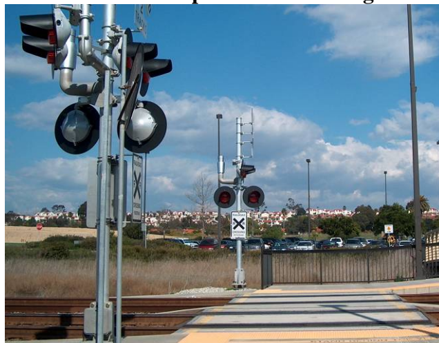
Figure 19. Flashing light signal assembly at an in-station pedestrian crossing
